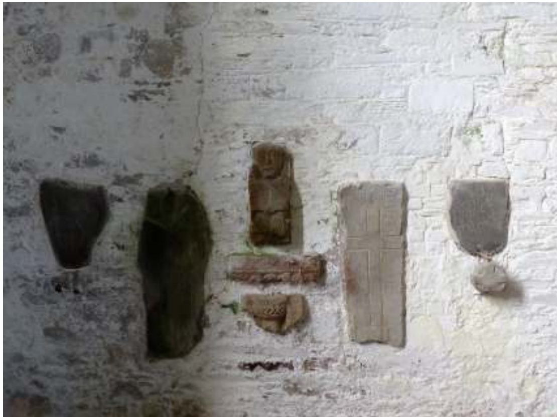
Fig. 1; Prior to works: the carvings had been set into the interior masonry wall with Portland cement, probably in the 1950s or '60s.
