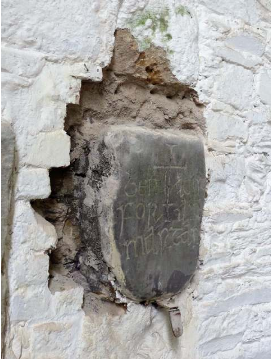
Fig. 3; Careful removal of surrounding masonry in order to safely extract the carvings.
